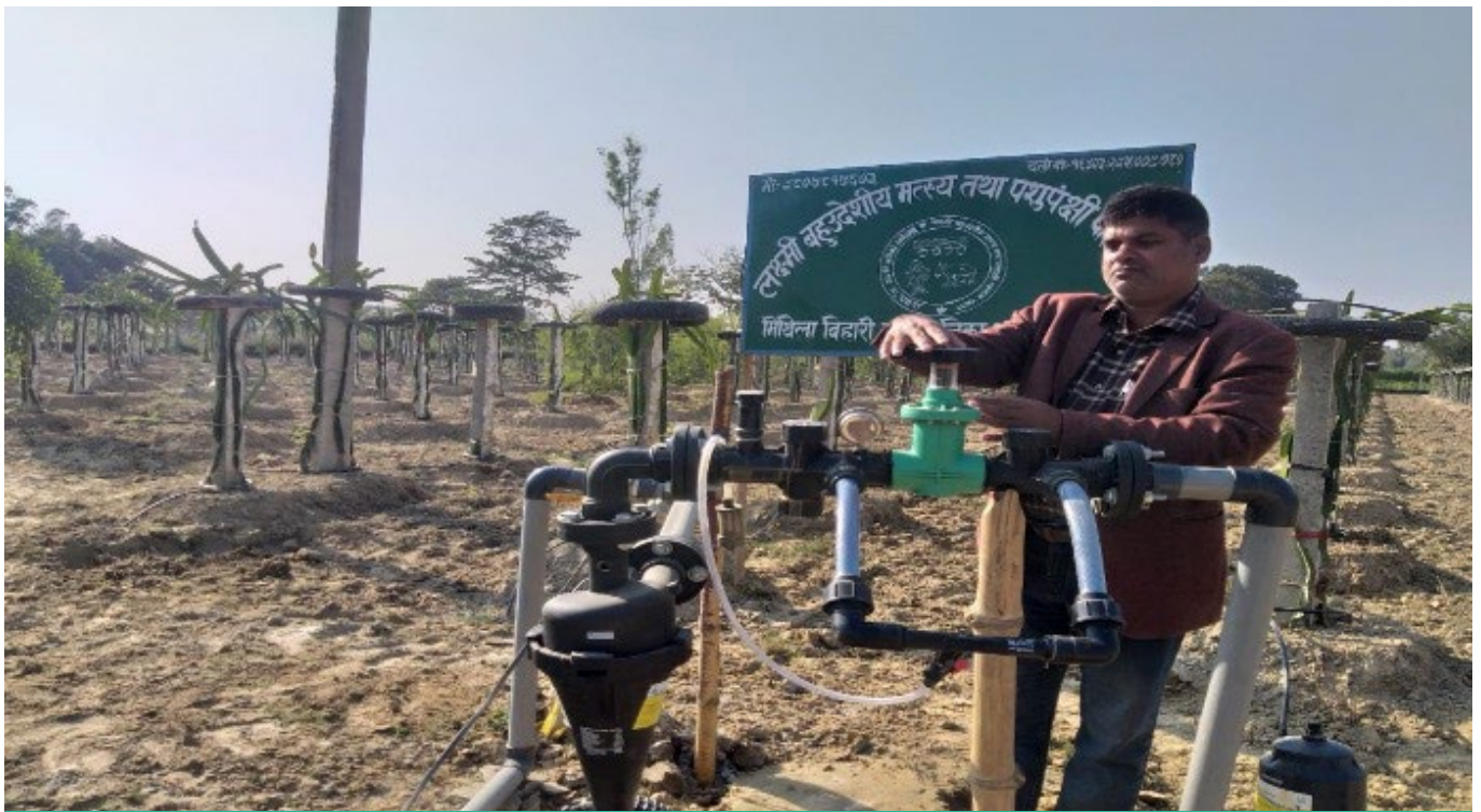
Image 5. Installation of Drip Irrigation System by Challenge Fund Grantee of Laxmi Bahuudeshya Matsya Tatha Pashupanchhi Firm in Dragon Fruit Farm at Mithila Bihari Municipality, Dhanusha
