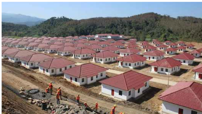
The houses constructed for families in Luang Namtha province who were displaced when the Laos-China Railway was built.
